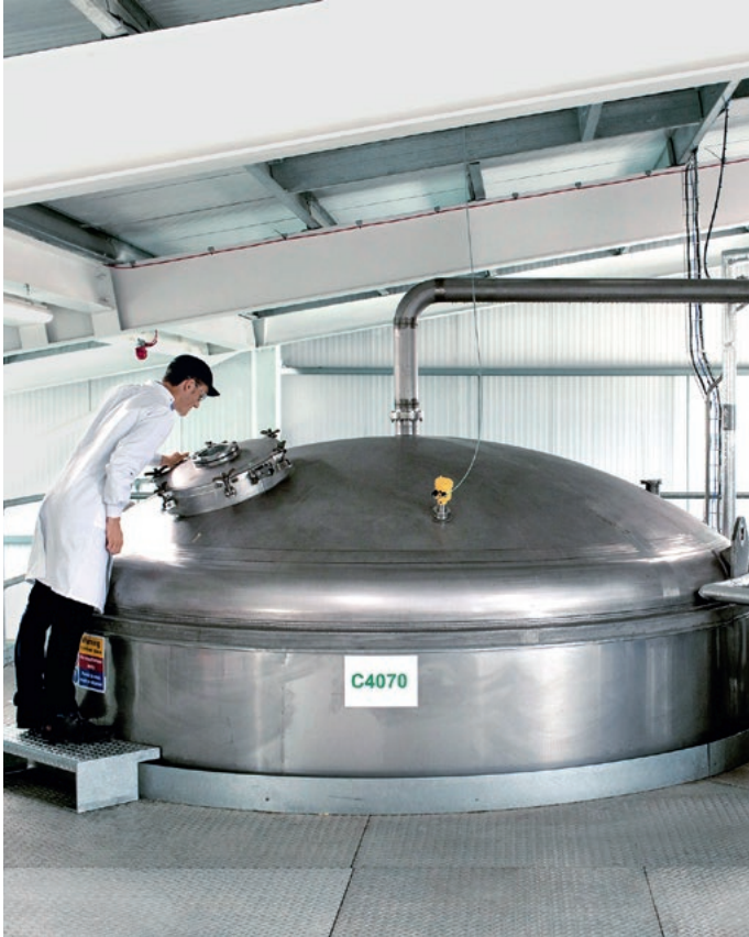
At its site in Littlehampton, BASF breeds nematodes in a 102,000-liter fermenter tank, spanning several levels.
